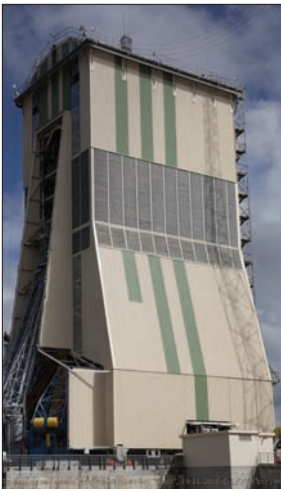
Construction is ongoing for the Soyuz launches in French Guiana. Photographer: Aleksey Yakunin.
